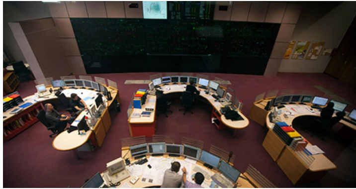
Figure 2: Control Room of the grid today
